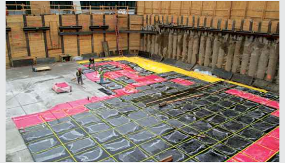
Building foundation bearings
