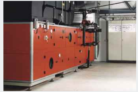
HVAC system installed in cellar
