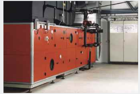
AC system installed in cellar
