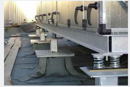
Roof-mounted HVAC system
