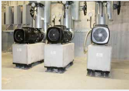
Bearing of pumps with additional mass
