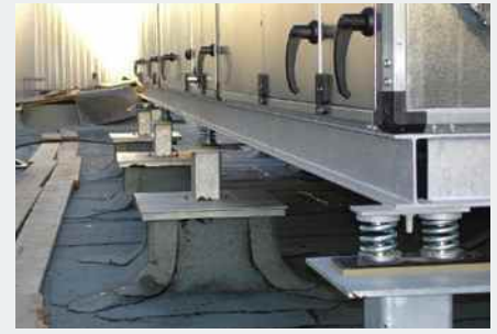
Roof-mounted HVAC system
