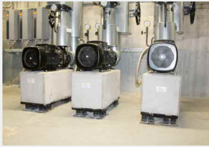
Bearing of pumps with additional mass
