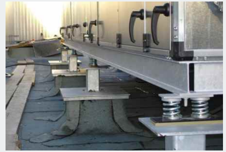
Roof-mounted AC system
