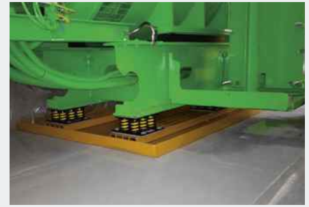
Large combined heat and power plant with several start-stop cycles
