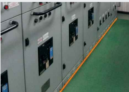
Decoupling of a power distribution unit on a service vessel
