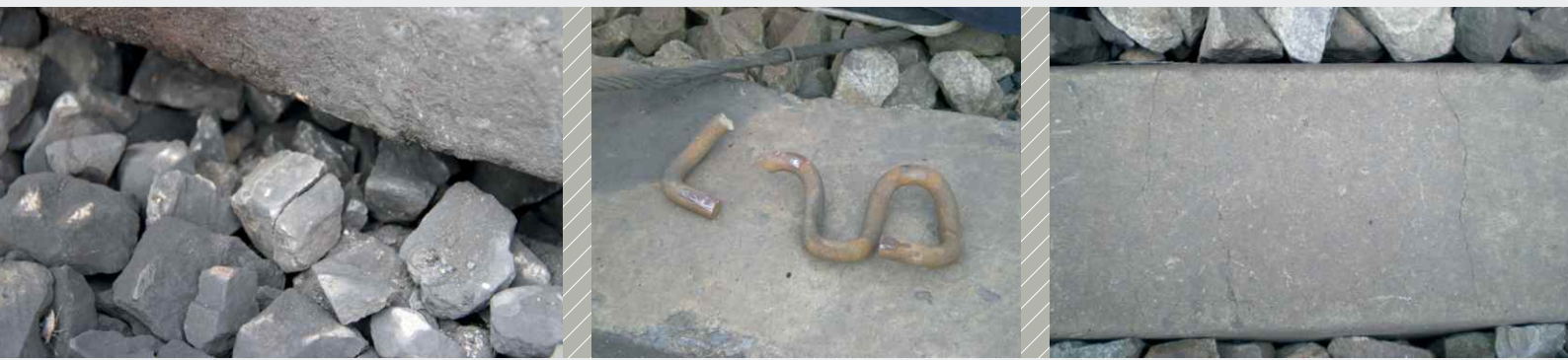
Destroyed ballast, rail clips and sleepers due to inhomogeneously embedded sleepers
