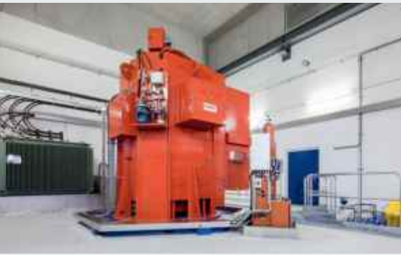
Elastic decoupling of the power plant
