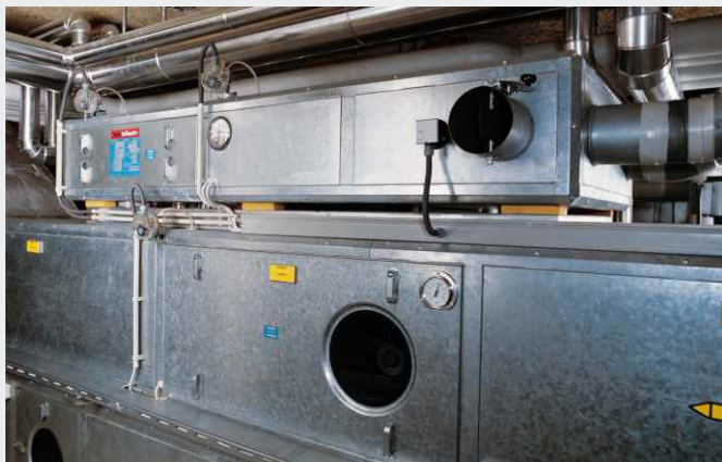
Decoupled air handling unit module
