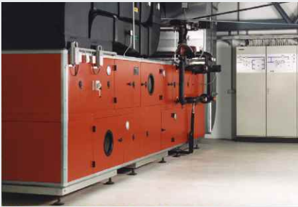
HVAC system installed in cellar
