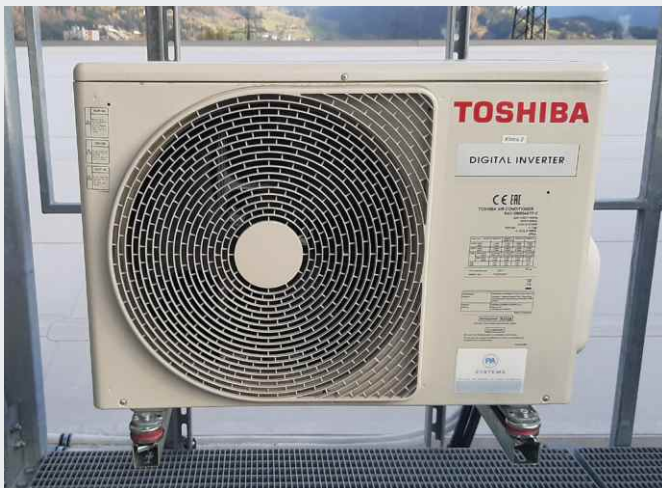
External air conditioning unit on wall bracket
