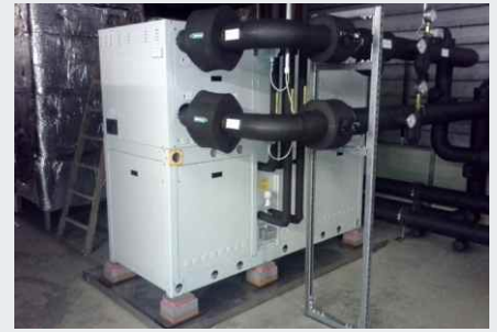
Chiller indoor unit
