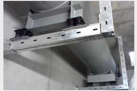
Bearing of duct silencer
