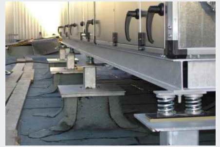
Roof-mounted HVAC system
