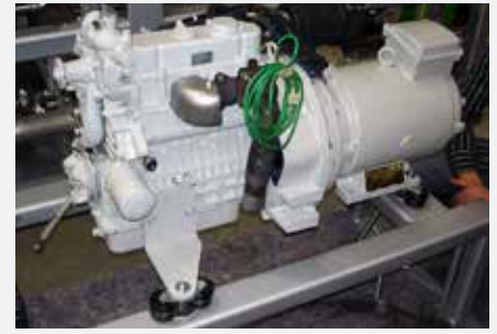
Small combined heat and power plant
