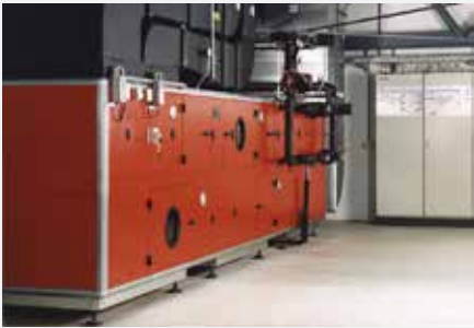
AC system installed in cellar
