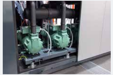
Industrial heat pump
