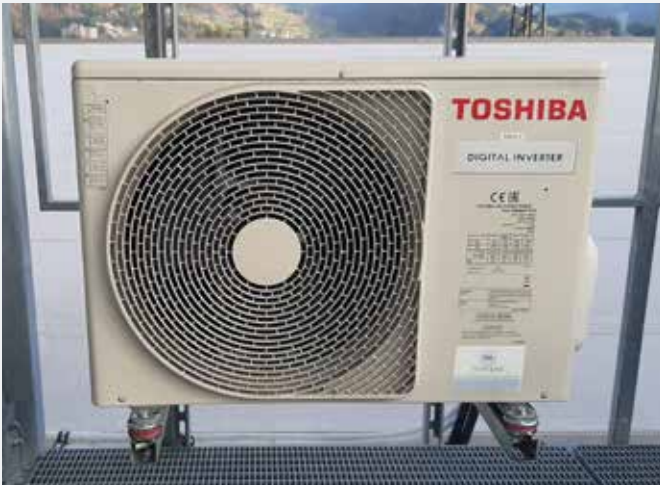
External air-handling unit on wall bracket
