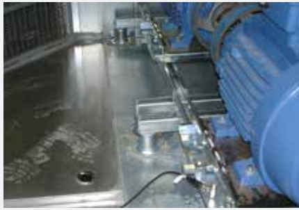
Bearing of belt-driven fans
