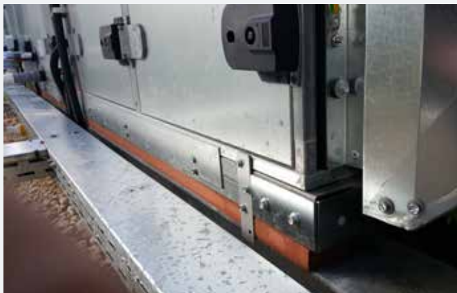
Strip bearing for air conditioning (AC) unit
