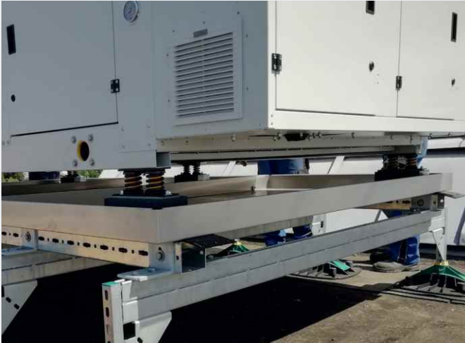
Unit installation in the drip tray
