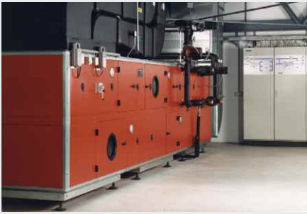
HVAC system installed in cellar
