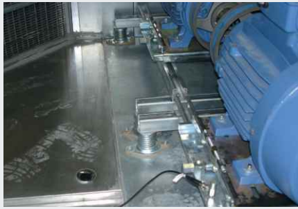
Bearing of belt-driven fans
