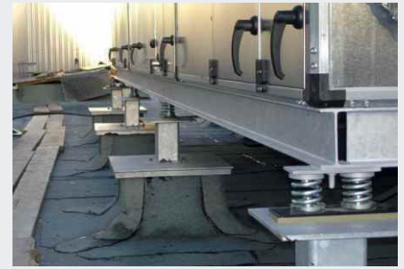
Roof-mounted HVAC system
