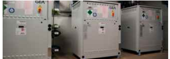
Effective bearing of refrigeration plant in the roof space
