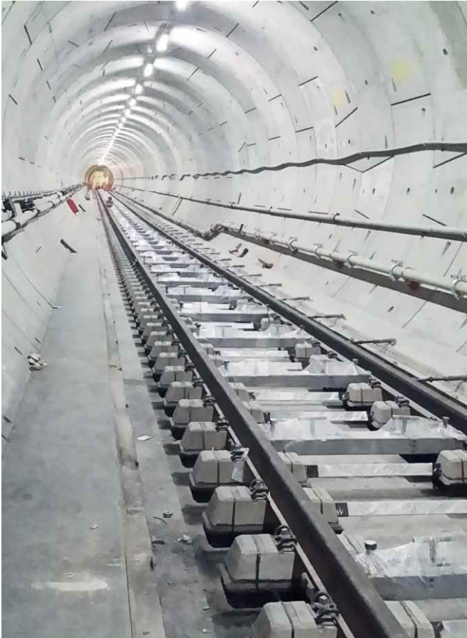
Slab track system in the tunnels
