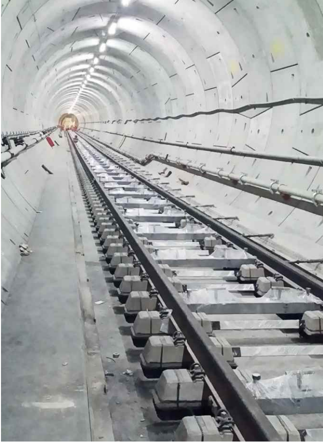
Slab track system in the tunnels
