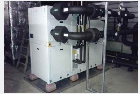
Chiller indoor unit
