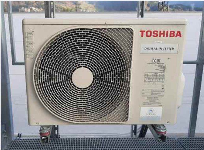
External air conditioning unit on wall bracket
