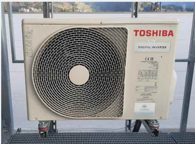
External air conditioning unit on wall bracket
