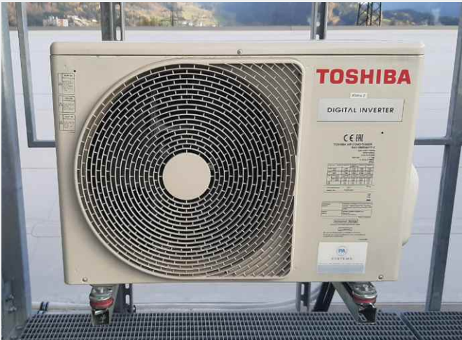
External air-handling unit on wall bracket
