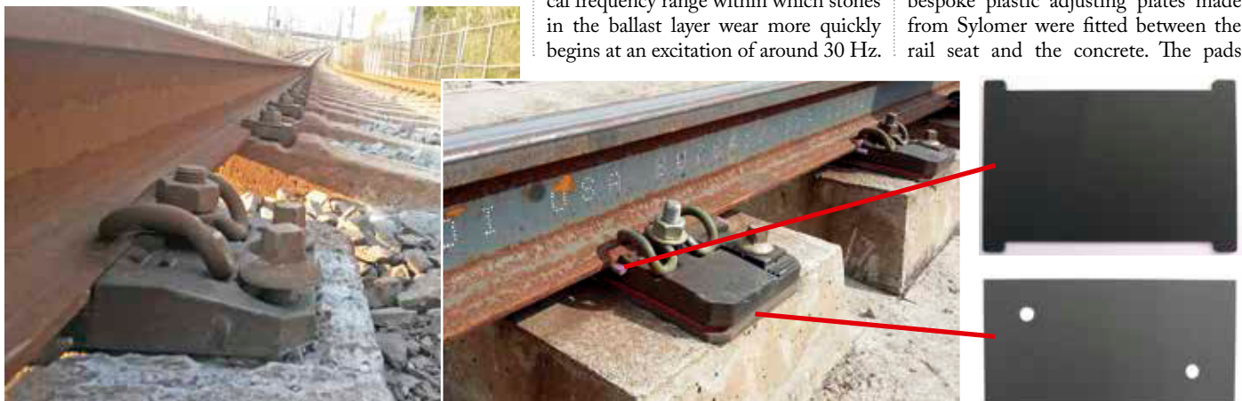
Fig 6. Damage to slab track with loosened fastening bolts (below) can be resolved by installation of plastic compensating plates and elastic rail pads (centre, right).
