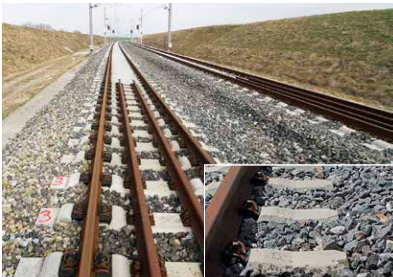
Fig 4. Guard rails along the transition (above). Bonding as a way of stabilising the ballast (right).
