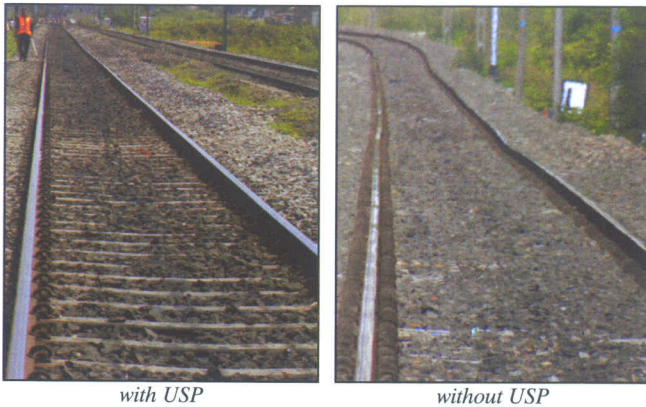
Fig. 9: Track with under-sleeper pads (left) and without (right)
