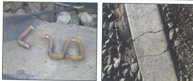
Fig. 1: White spots – an indication of ballast destruction (top), broken rail clips (left) and sleeper cracking (right), resulting from excessive dynamic traffic loading
