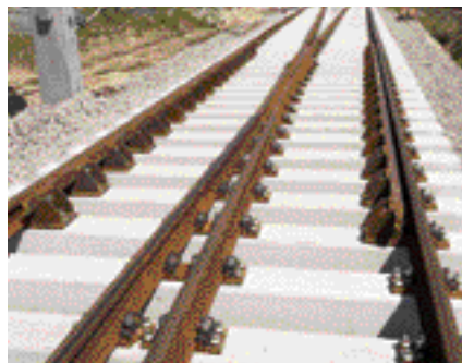
Turnout with rigid crossing frog and check rails
