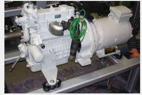
Small combined heat and power plant
