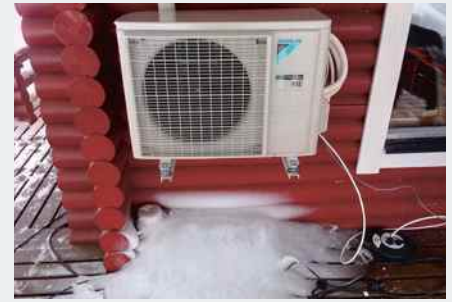
External unit of a heat pump on a wall bracket
