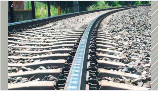
Rail with corrugation
