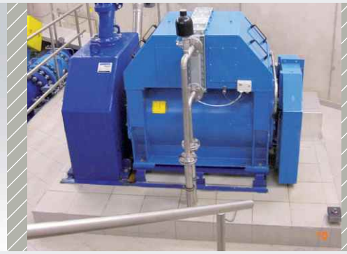
A pleasant working environment close to turbines
