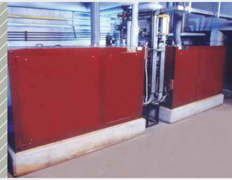
Elastically mounted combined heat and power plant
