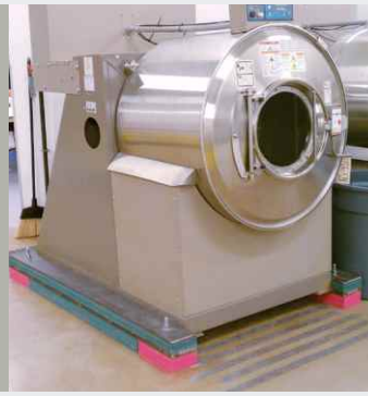
Elastic decoupling of an industrial washing machine
