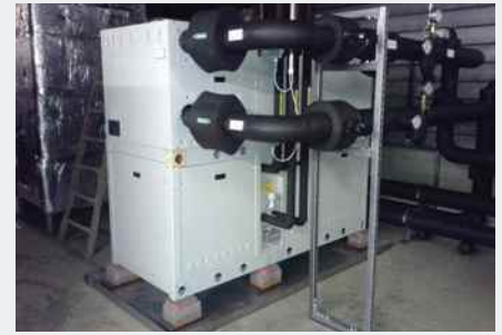
Chiller indoor unit
