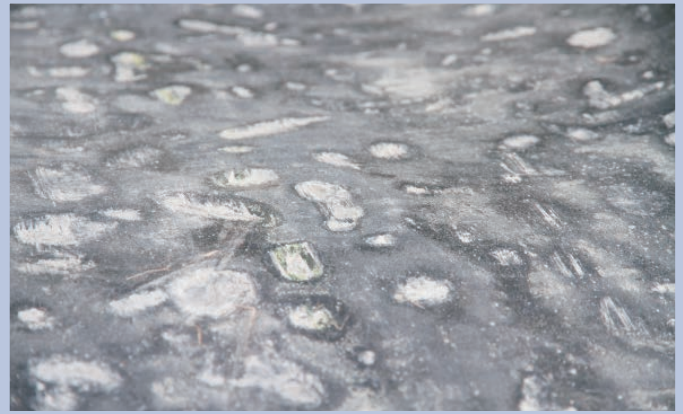
Fig. 3: Removed ballast mat showing indentations from ballast stones
