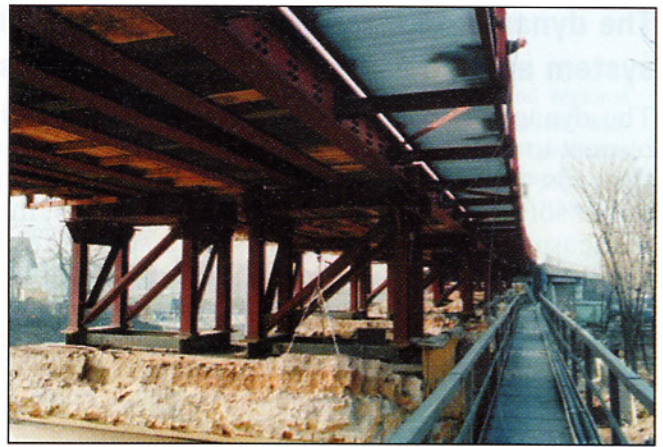
Fig. 6: Underside of the auxiliary railway bridge, which has been installed on top of the viaduct segments (Photo: W. Weißenberger, Müller-BBM)
